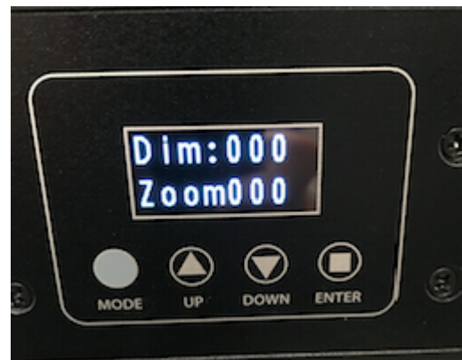
NO DMX CABLE CONNECTED
