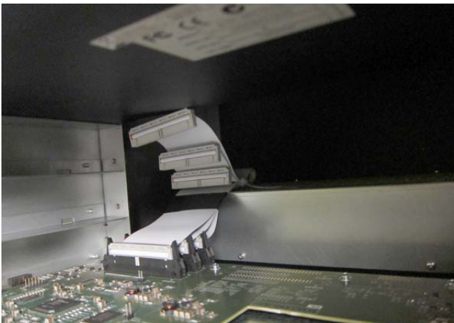
Figure 20. I/O card ribbon cable bundle (front view)
