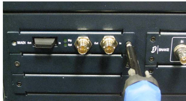
Installing the MADI card in the FOH Rack
